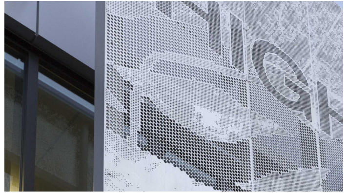
PERFORATED METAL SIGNAGE FOR HIGHLAND PARK COMMUNITY CENTER. PHOTO © CHRISTIE RACHELLE.
